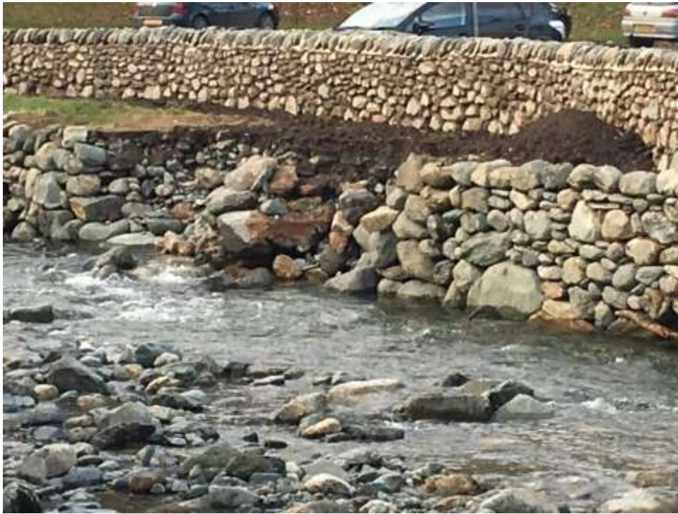
Fresh beck wall collapse above TIC
